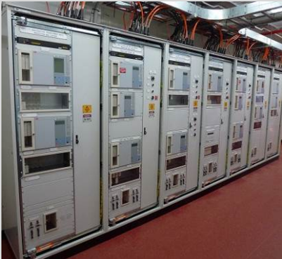
Substation Automation – IEC61850
